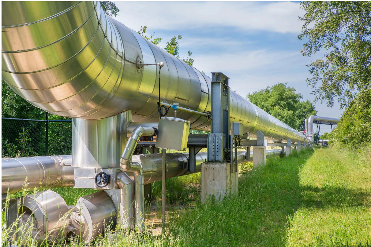
Large gas pipeline. Source: Adobe Stock.
